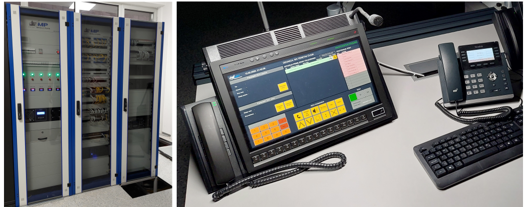
Figure 12. On-site deployment of the digital dispatching system, showing rack-mounted central equipment and dispatcher TC desk, illustrating practical integration of software-centric services within an operational railway environment.
